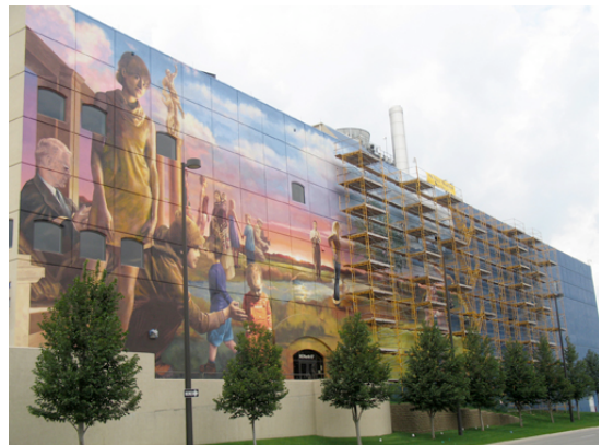
The first section of scaffolding came down this week as work continues on Fertile Ground the Omaha Mural Project. Photo: Holly McAdams
